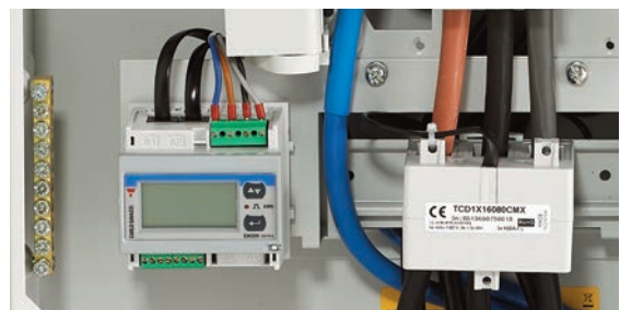
One dual channel standard meter (via two separate block CTs) for separate lighting and power readings
